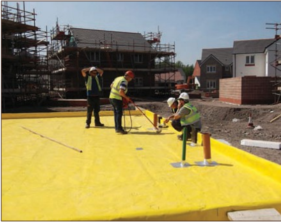
Figure A4.43 Dielectric porosity testing for housing scheme (courtesy NHBC)
