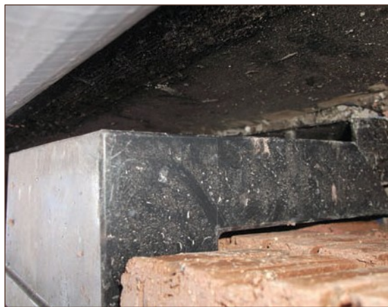
Figure A4.88 Ventilator becoming detached to fit to external block work. This is due to builders requiring increased cavity widths to achieve thermal properties expected by Building Regulations (courtesy NHBC)
