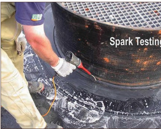
Figure A4.45 Spark testing (courtesy GSE Environmental)
