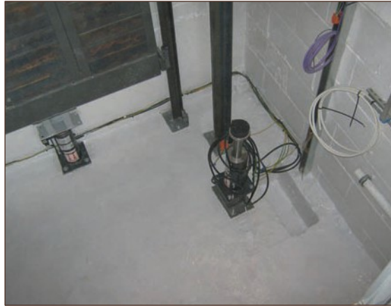
Figure A4.32 High quality installation of liquid gas membrane to lift pits, including resin gas protection on all screw penetrations (courtesy Card Geotechnics Limited)
