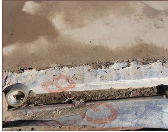
Figure A4.56 Gas membrane at edge of concrete screed. Screed has been grinded to achieve desired levels, gas membrane shows extreme wear and damage as a result (courtesy NHBC)
