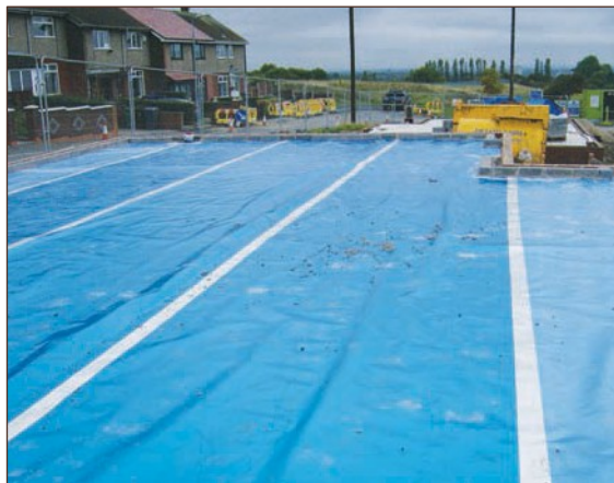
Figure A4.60 Some stones could penetrate gas membrane if sufficient force is applied (courtesy Smith Grant)
