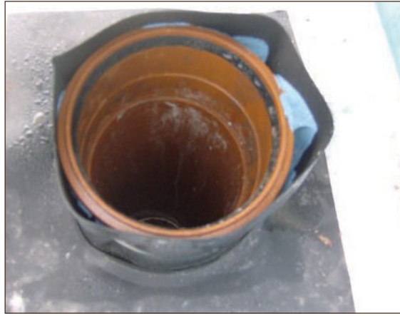
Figure A4.74 Gap between OD of service pipe and ID of top hat too large: cannot be compressed enough to form seal, even with the application of additional tape (courtesy Smith Grant)
