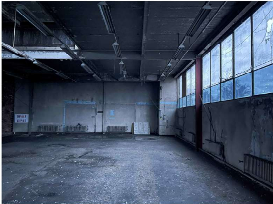
Above: Existing First Floor, with Partial Boarded Windows
