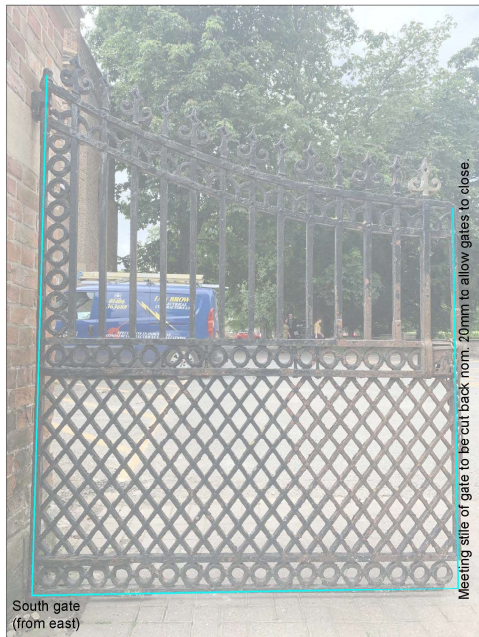
View of gates from east (inside Ayscoughfee Gardens) - showing visible defects and repairs
