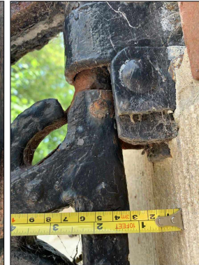
Fixed hinge point on south pillar Note: Fixed hinge does not allow for any realignment of the gates so they cannot be pulled out at the top to prevent clashing at the meeting stiles.
