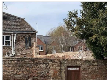
View of wall from SE after partial collapse and rebuild
