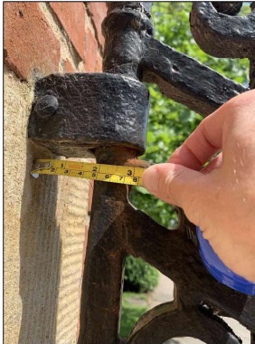
Fixed hinge point on north pillar Note: Fixed hinge does not allow for any realignment of the gates so they cannot be pulled out at the top to prevent clashing at the meeting stiles.
