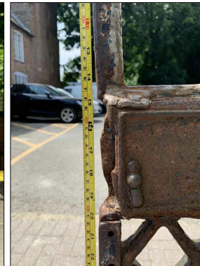
Lock box meeting stile - North gate Note: Lockbox damaged and gate frame badly distorted.
