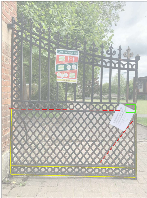
View of gates from west (the Chestnut Avenue) - showing visible defects and repairs
