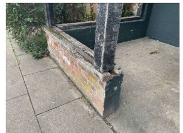
Image prior to works showing rotten timber plates
