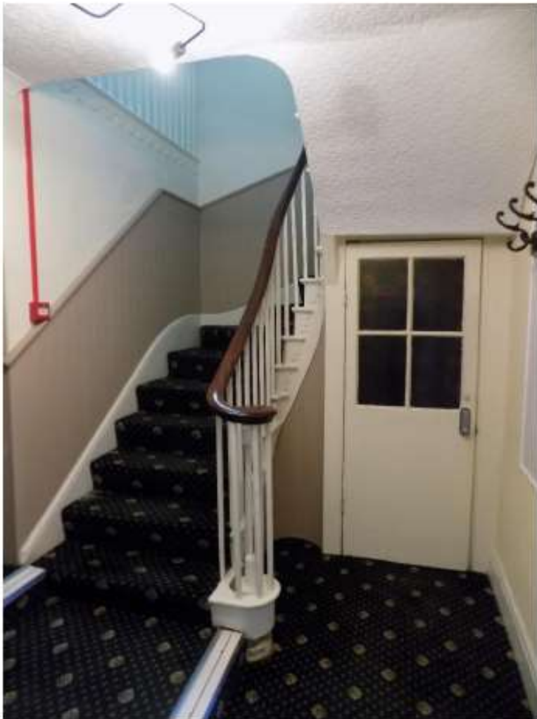
P19 – early 19 th century stick baluster staircase. Note the unusual arrangement with a stone under the wreath (used to lift a re-used staircase to the level required?)
