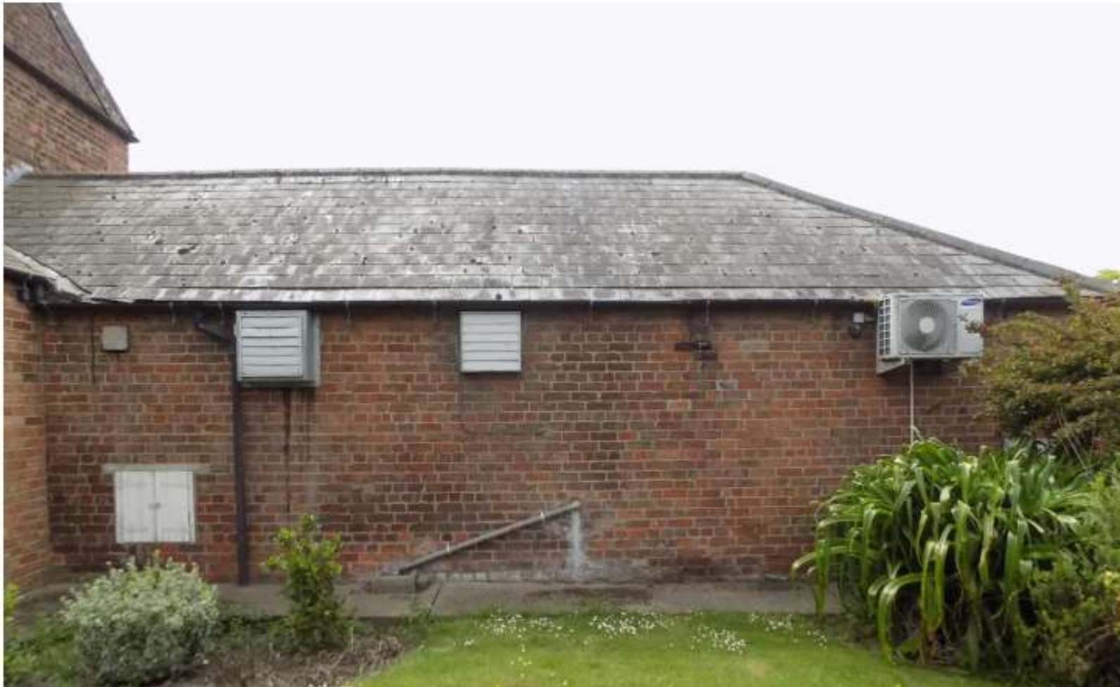
P4 – east elevation of stable. The modern requirements of a commercial kitchen detract from the exterior.
