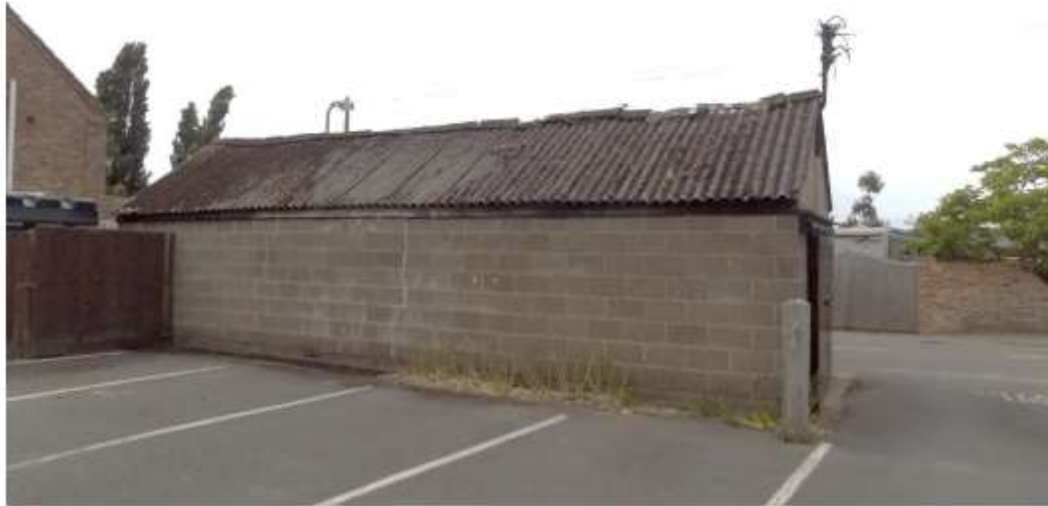
P11- south elevation of store - concrete block and a corrugated iron roof.
