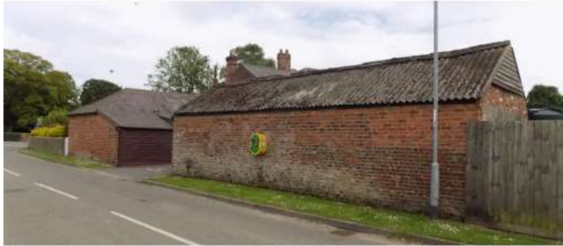
P10 – north elevation of Store- contains old brickwork at the lower level.
