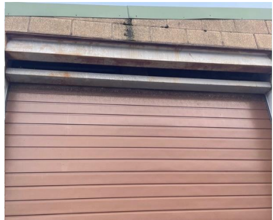
Photograph 13: Gap above the roller door
