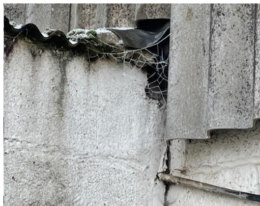
Photograph 17: Gap where block room joins the main building
