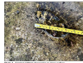
Photo 4 - Nominal 110mm depression in stone surface
