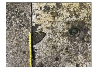
Photo 7 - Nominal 50 to 100mm depressions in stone surface
