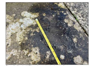
Photo 6 - Nominal 250mm depression in stone surface
