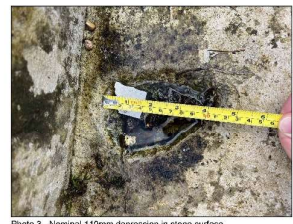
Photo 3 - Nominal 110mm depression in stone surface
