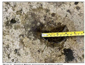
Photo 2 - Nominal 80mm depression in stone surface
