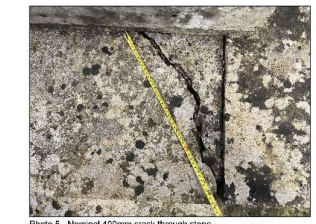
Photo 5 - Nominal 400mm crack through stone
