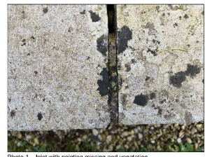
Photo 1 - Joint with pointing missing and vegetation
