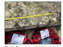
Photo 8 - Depressions and damaged joints to stone
