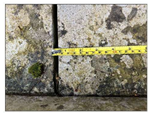
Photo 11 - Algae growth on stone surfaces, pointing missing
