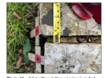
Photo 10 - Joint with pointing missing / eroded
