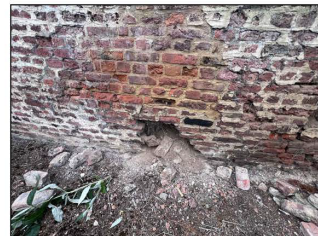
Detailed view Area of collapse A
