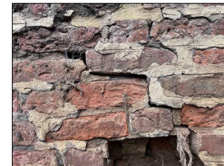
Detailed view Cracking above area of collapse B
