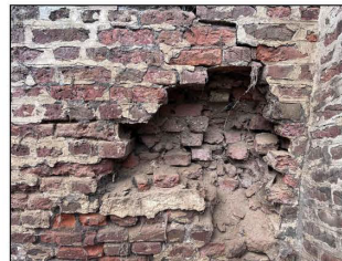
Detailed view Area of collapse B
