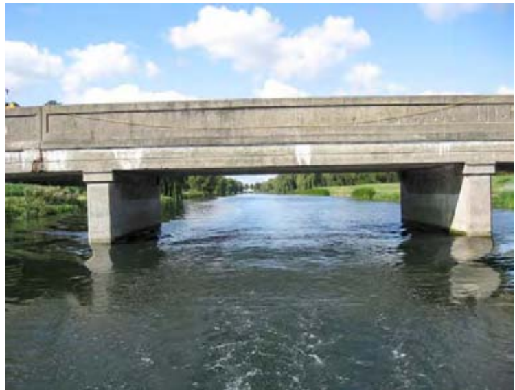
Low bridges on the Coronation Channel will prohibit navigation by craft constrained by their 'air draught'. As a long-term aspiration bridges should be raised to allow navigation
