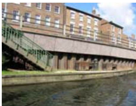
The restoration of old wharves provides an opportunity to create a positive river frontage
