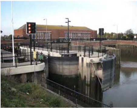
The completed Black Sluice Lock forms a 'Gateway' onto the Black Sluice Navigation, Boston
